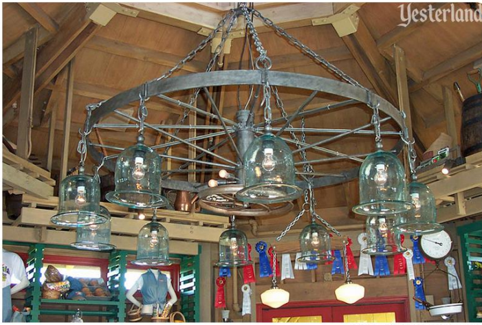
Overhead light fixture
